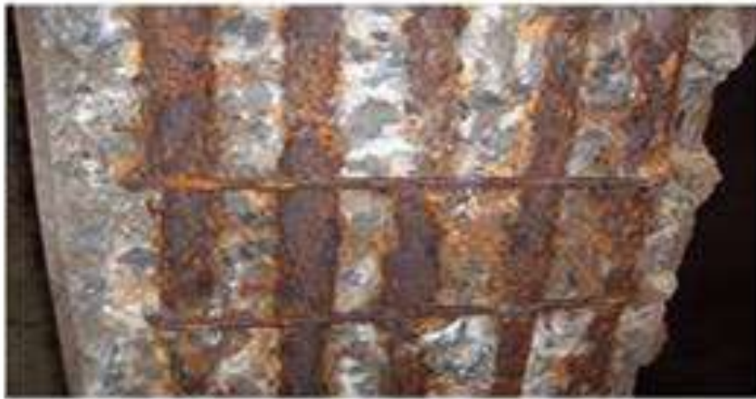
Fig.2 Corrosion in RC structure
